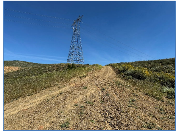
Transmission line corridor
